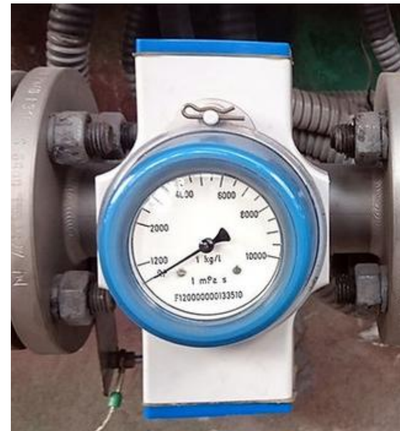
Water submeter systems in apartments and common areas help identify leaks to reduce waste and expenses
